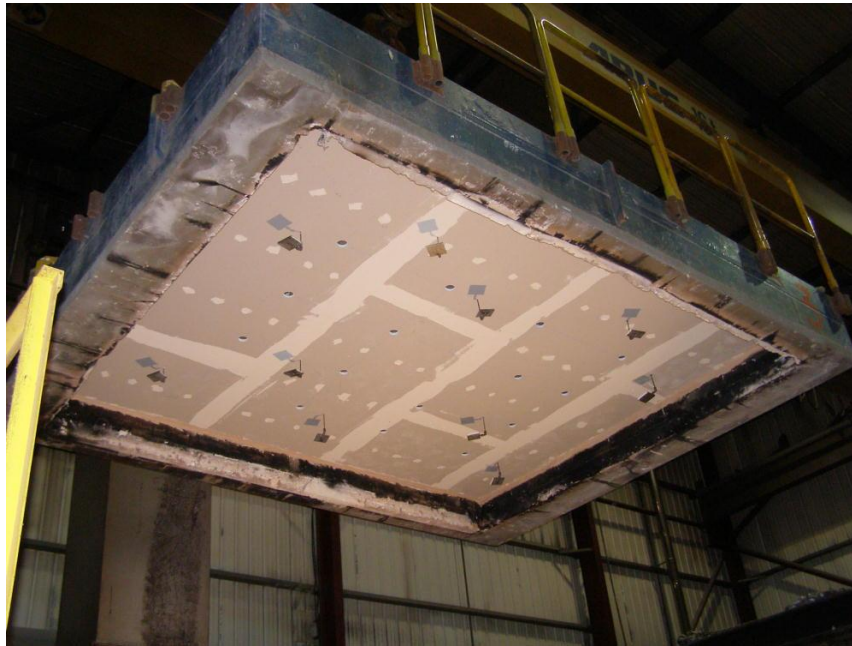
Plate 1 Test construction being lifted onto furnace before test, showing holes drilled in ceiling prior to installation of downlights.
